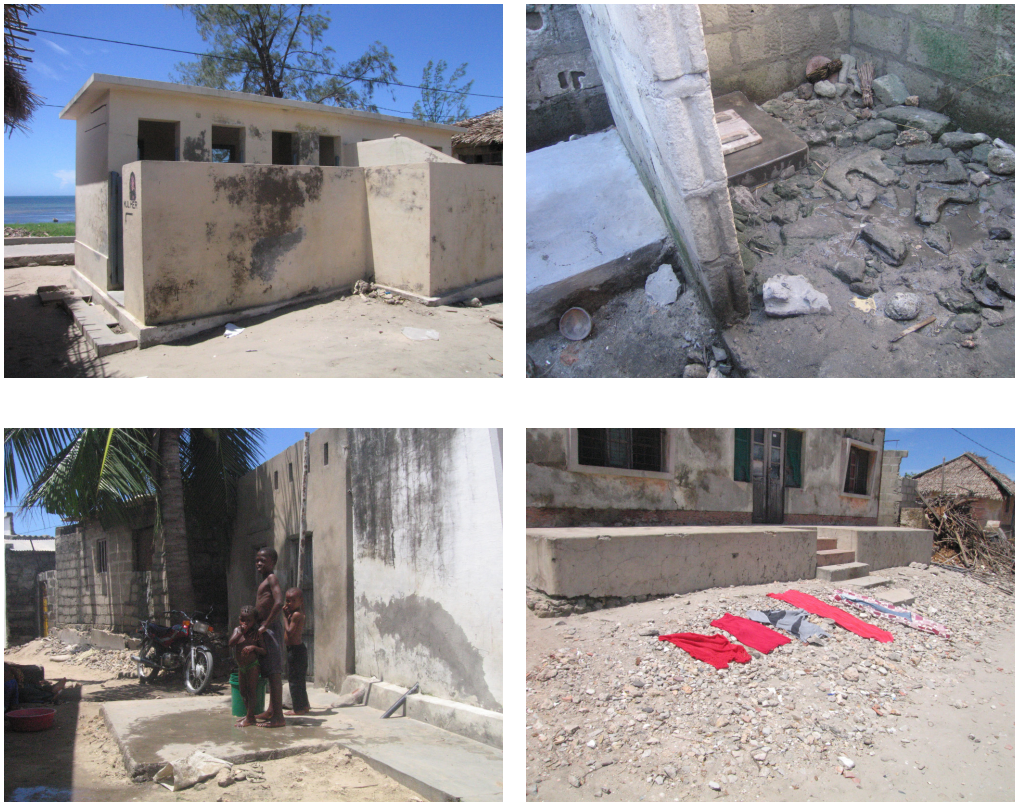
Figure 16: Public and private sanitation facilities
