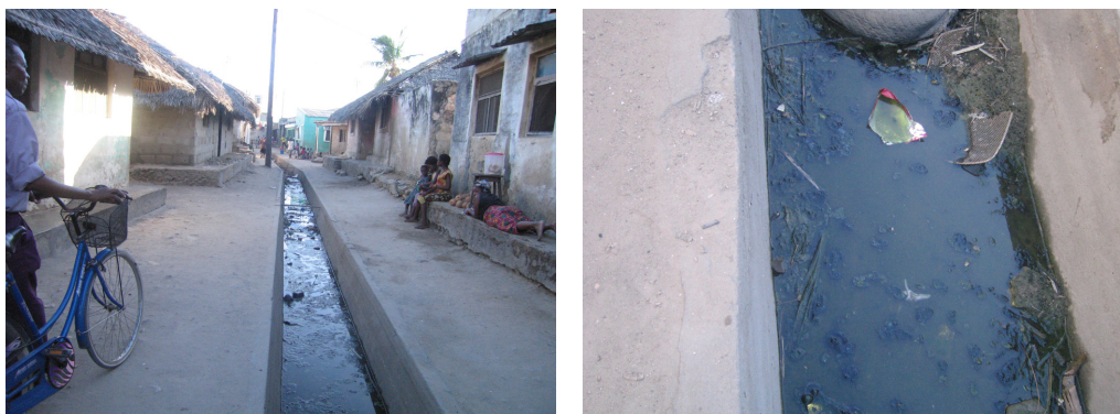
Figure 17: Open drainagen in Macuti Town
